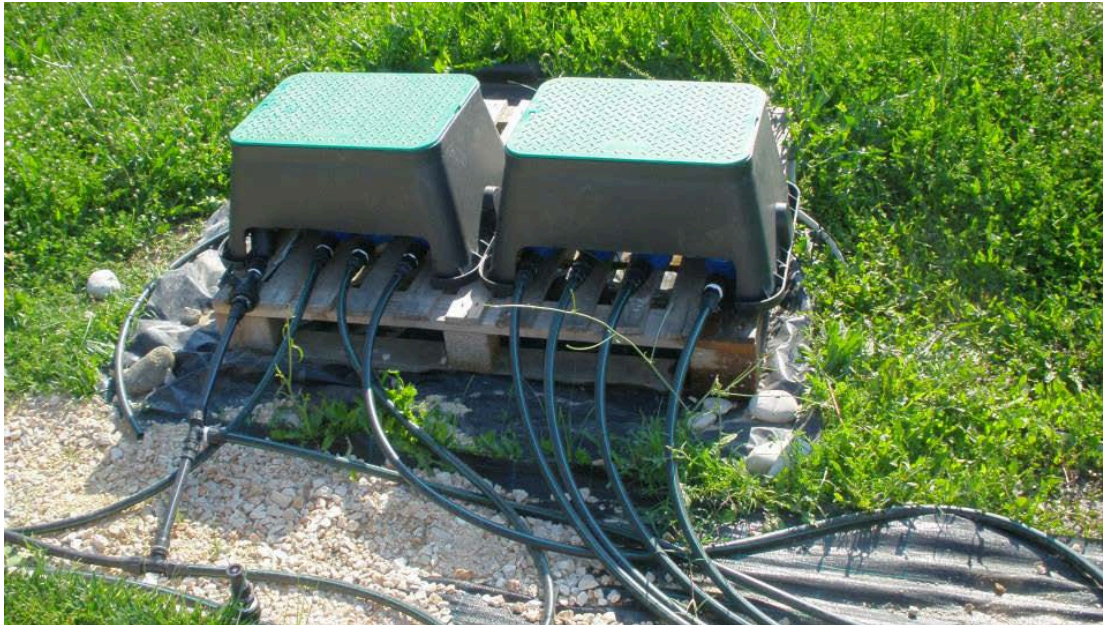
Fig. 20 Control valve boxes
