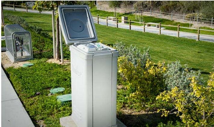
Fig. 9 Professional irrigation controller housed in special waterproof security box
