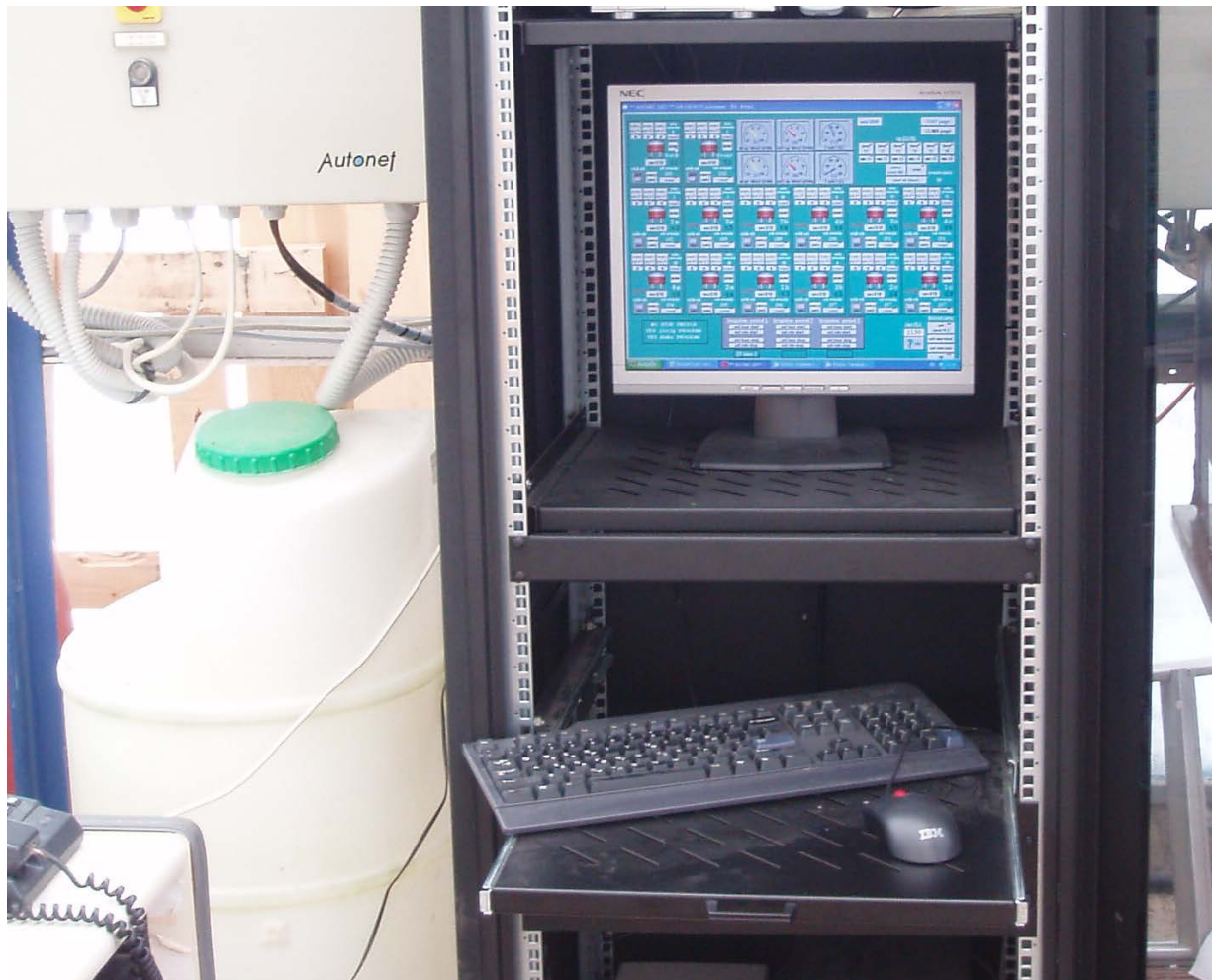
Fig. 6 The automation of irrigation in the experimental greenhouse of TEIEP
