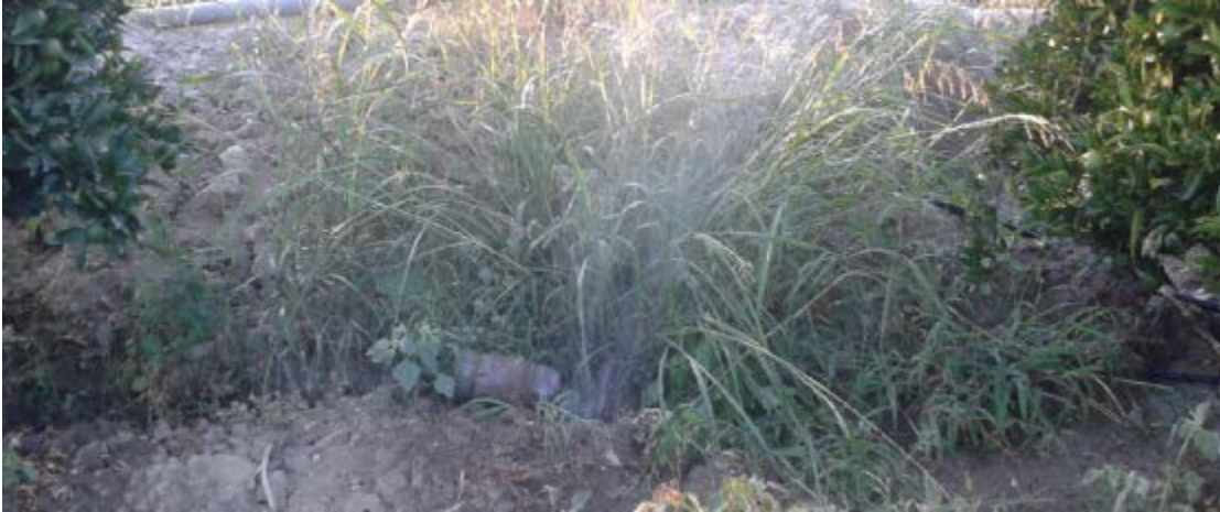
Fig. 44 Leakages in irrigation pipes (main pipe)
