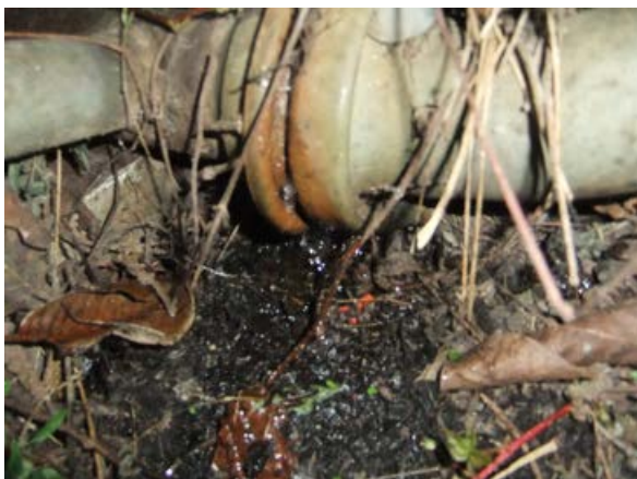
Fig. 57 Irrigation problems in greenhouses (leakages in irrigation pipes)
