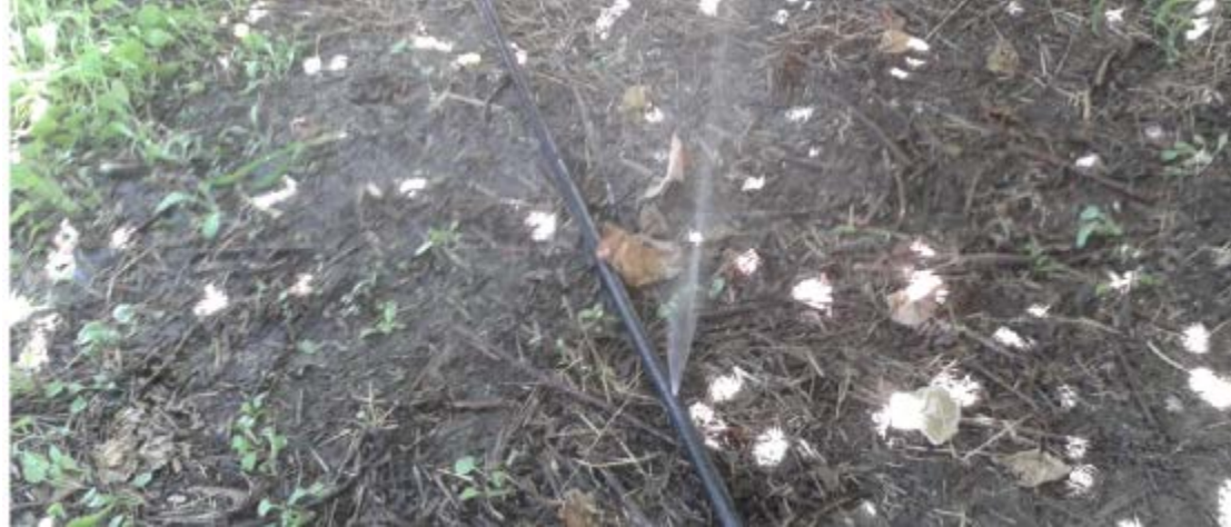
Fig. 46 Leakages in irrigation pipes (tertiary pipes)
