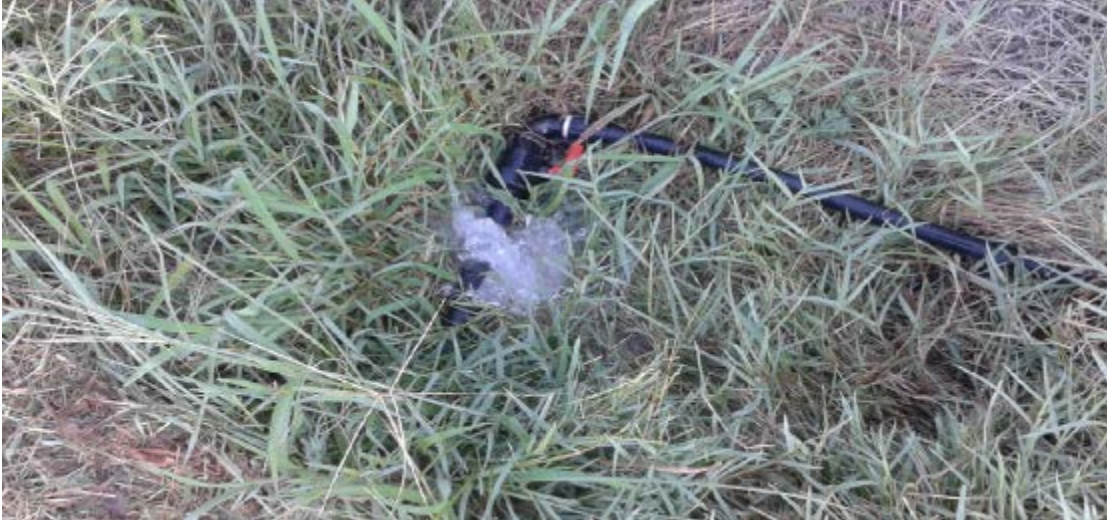
Fig. 45 Leakages in irrigation pipes (secondary pipes)
