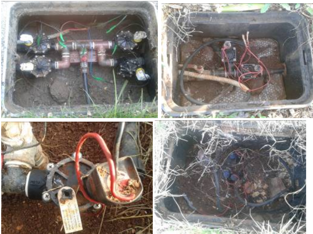
Fig. 62 Control valves in study landscapes
