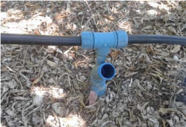
Fig. 47 Total absence of filter in junctions
